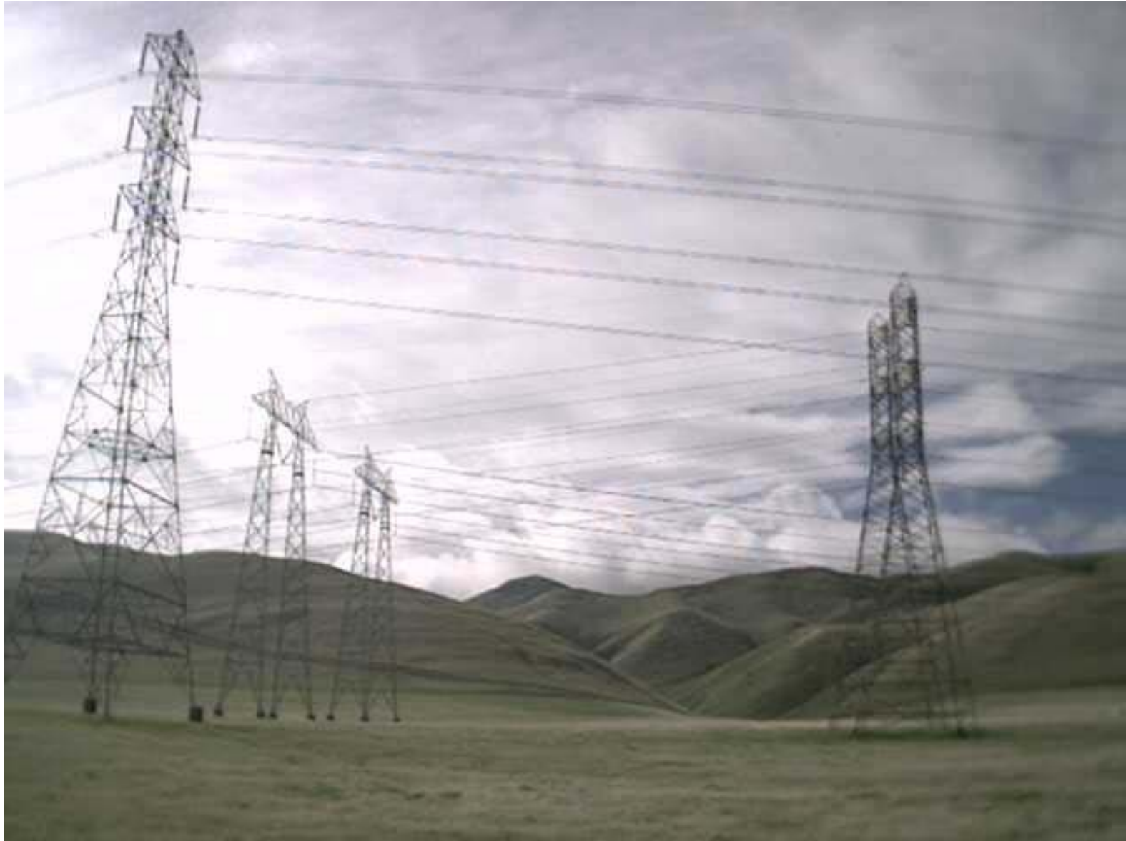
POWER TRANSMISSION CORRIDOR VIEW WEST – 8 CIRCUITS
