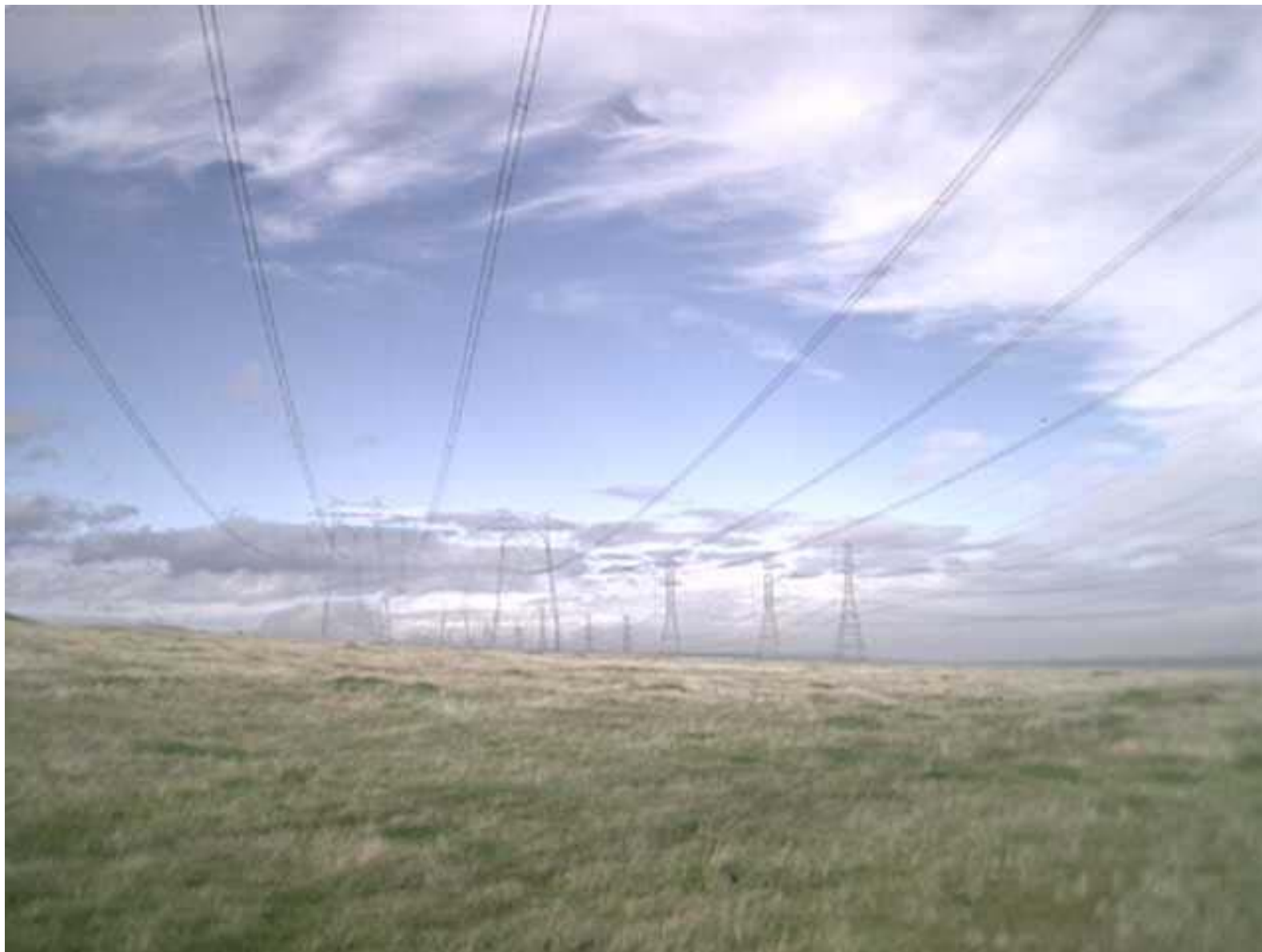
POWER TRANSMISSION CORRIDOR VIEW NORTH – 8 CIRCUITS
